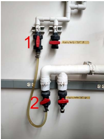
Figure A1. Bypass valves in open positions.
